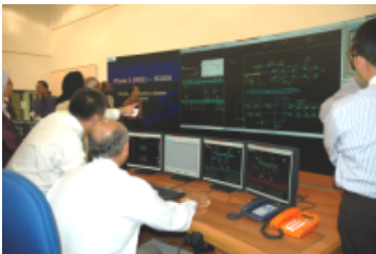
Picture-3: Metro Regional Control Center
